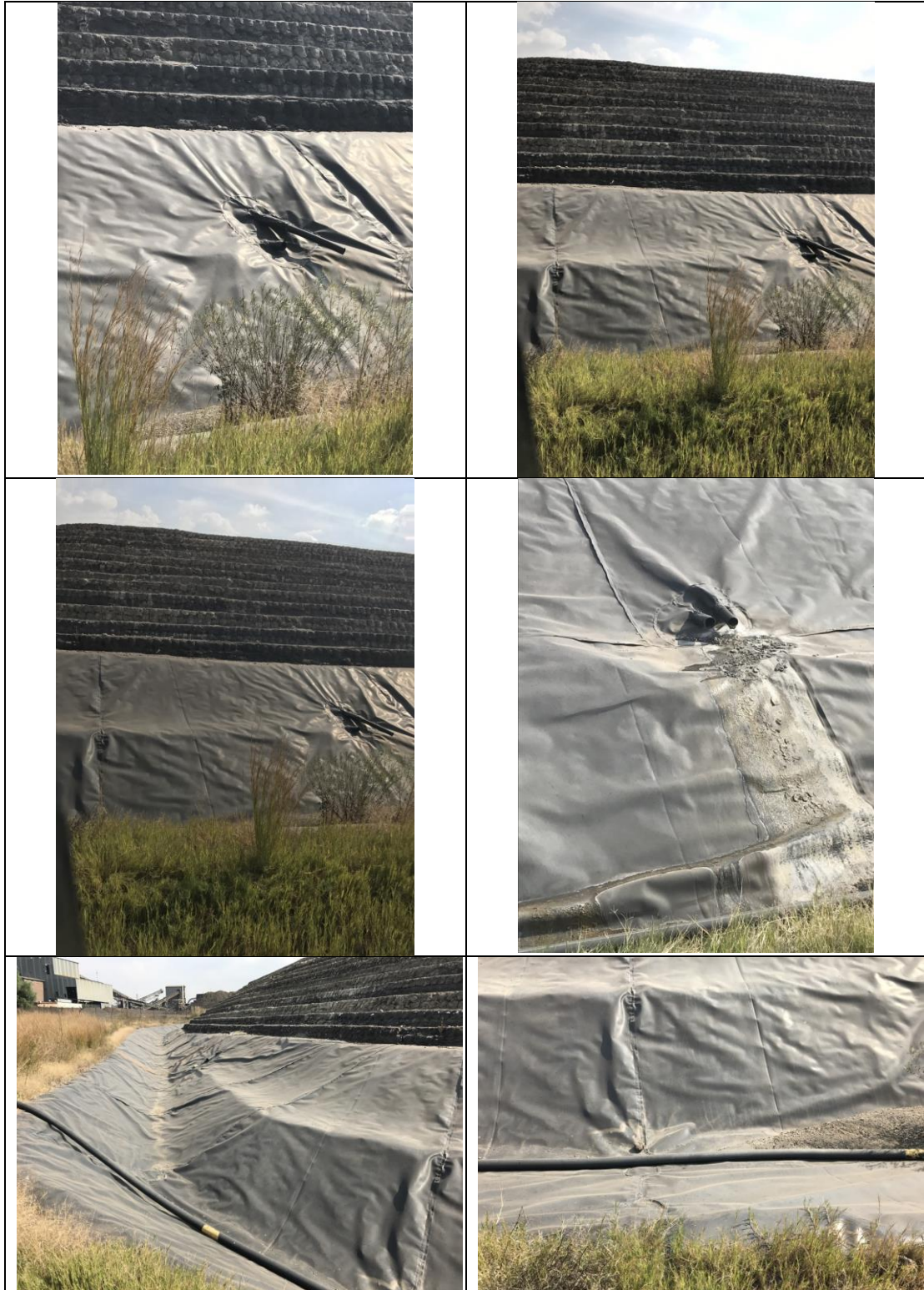
Showing plastic liner, drainage from WDF and storm water drainage along toe of WDF in a trench
