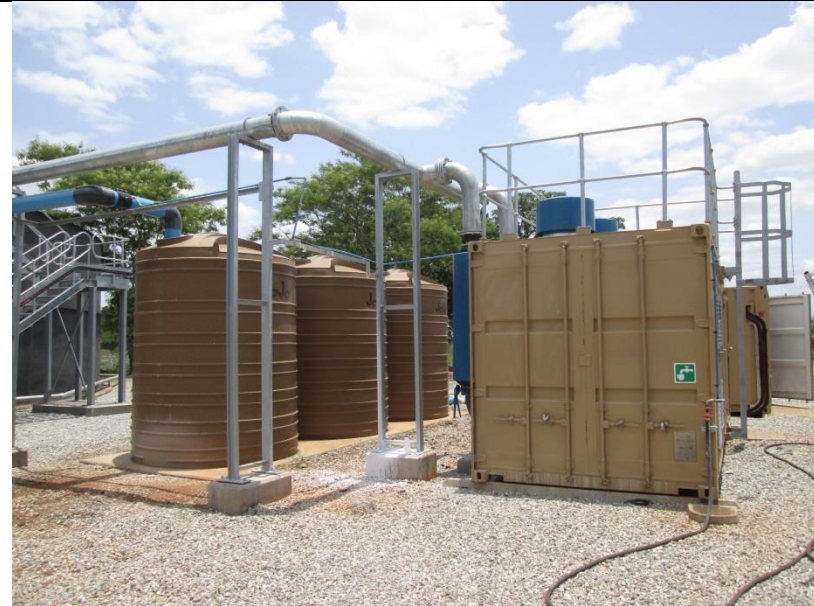
Photo 3: View of the existing package plant showing the infrastructure that will be decommissioned as part of the WWTW upgrade.
