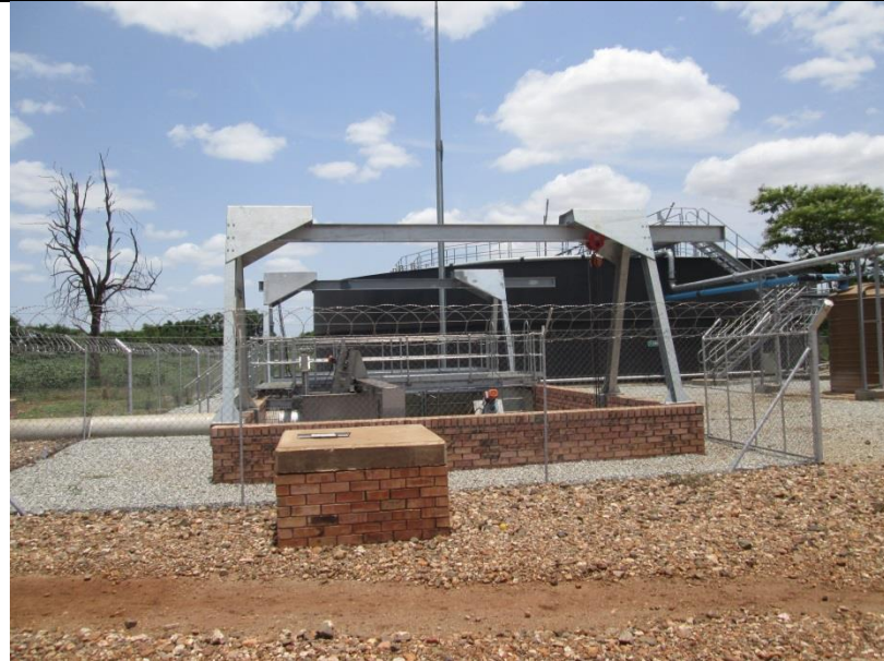
Photo 4: overview of the existing package plant, showing water retention dam and inlet works
