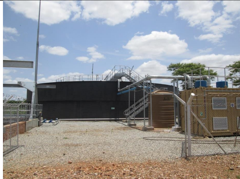
Photo 5: Overview of the existing package plant, showing treatment works and water retention dam.
