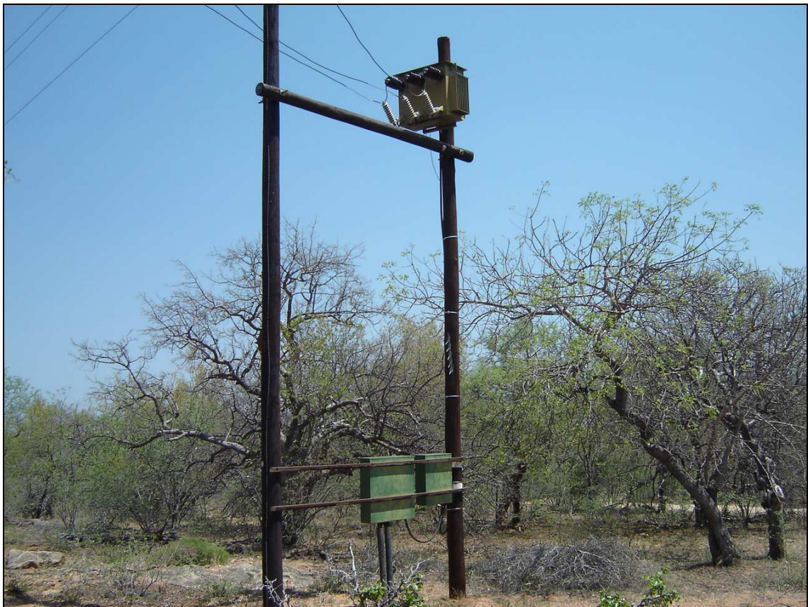
Figure 10: Eskom transformer on site
