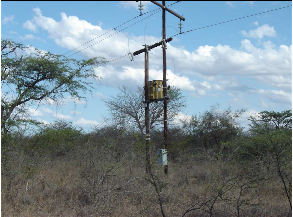
Figure 10: Eskom electricity is available on site
