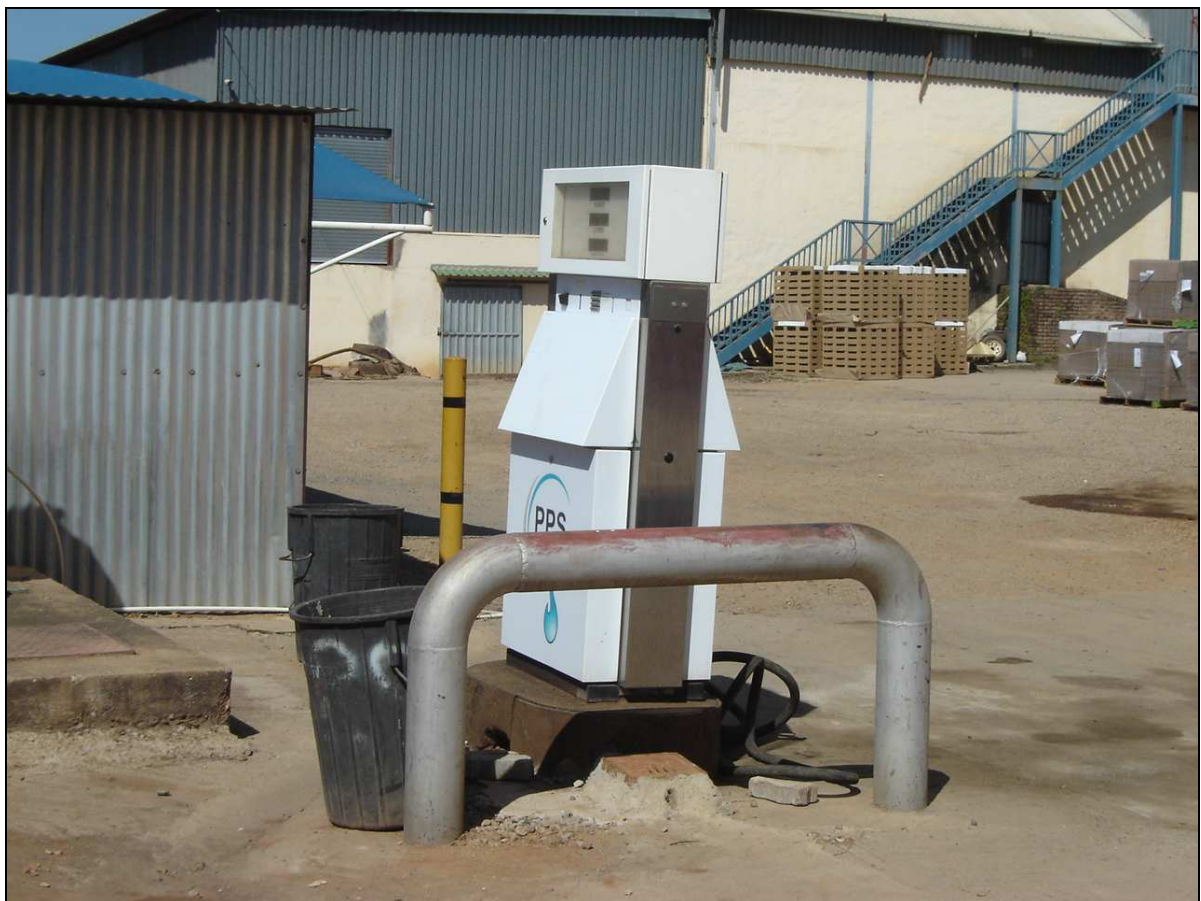
Figure 12: Existing pump on site
