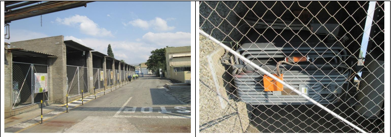
9 – Redundant Transformers: Looking in a Westerly direction from the centre of the site being demolished
