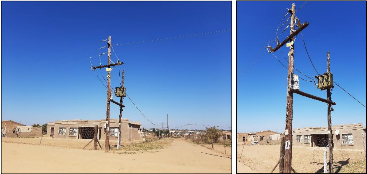
Images 3: Typical MV & LV electricity reticulation networks & step down transformers.
