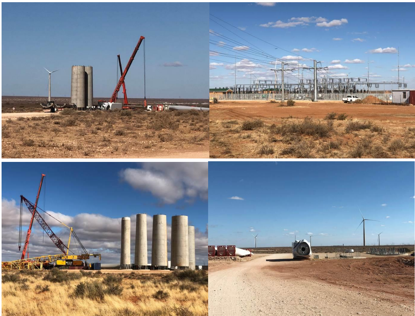
Figure 2-5: Photographs depicting the construction phase of a wind farm similar to Botterblom WEF.
