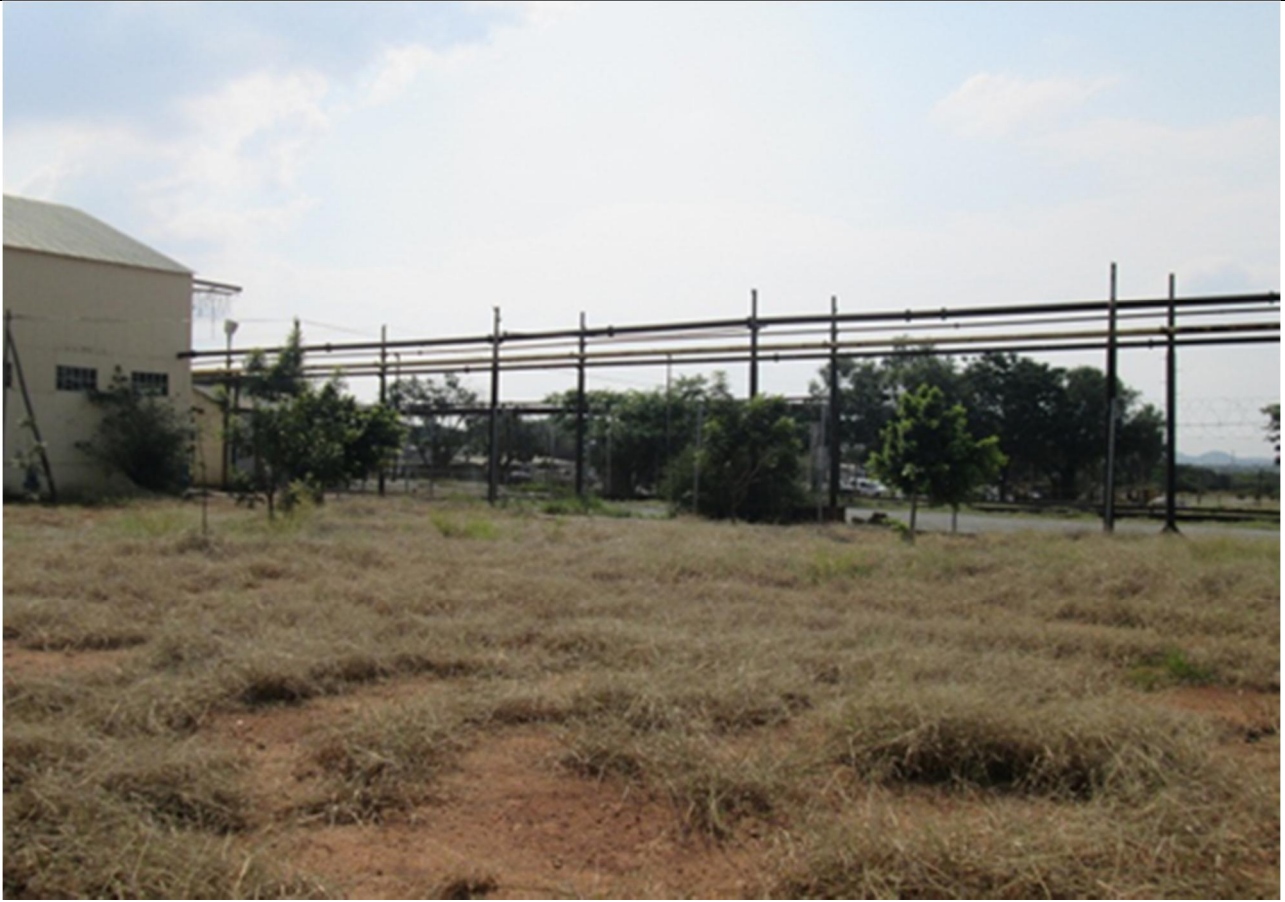
A Pipeline to the Thickener
