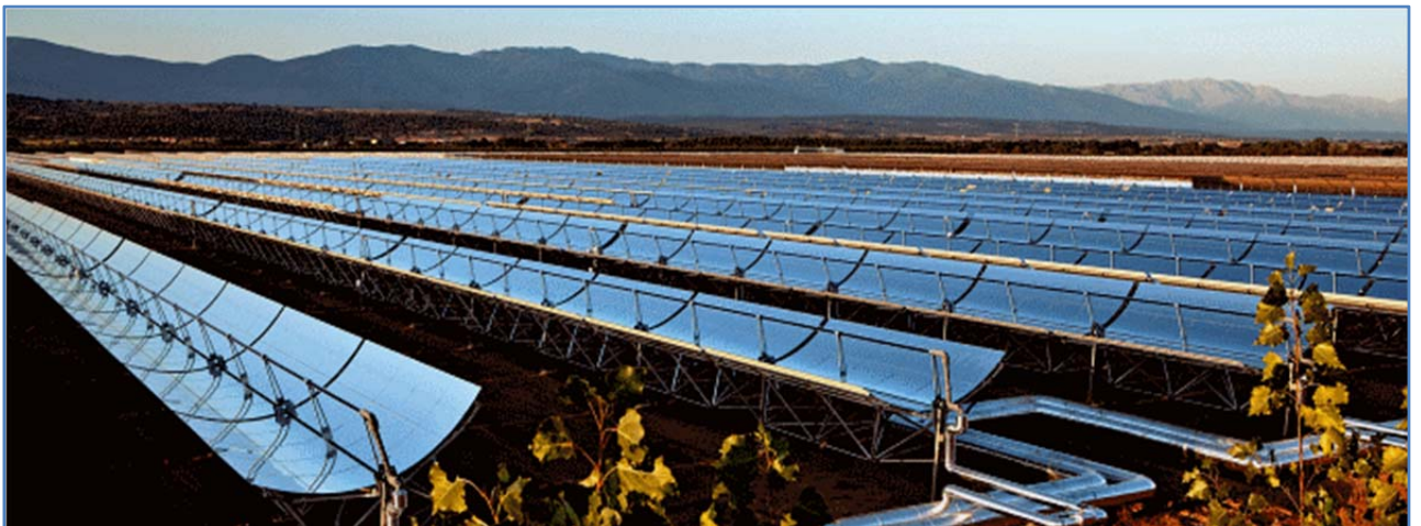
Figure 2: Example of a Concentrated Solar Power Parabolic Trough Facility
