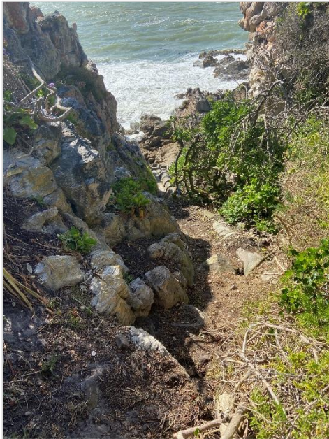
Figure 3: Western entry to proposed connection path for Alternative 1 over old stormwater pipe down the gully next to Erf 12257
