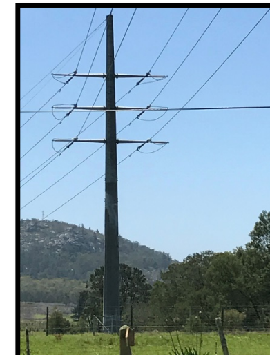
Photo 4: This photo shows a typical 132kV monopole powerline route.
