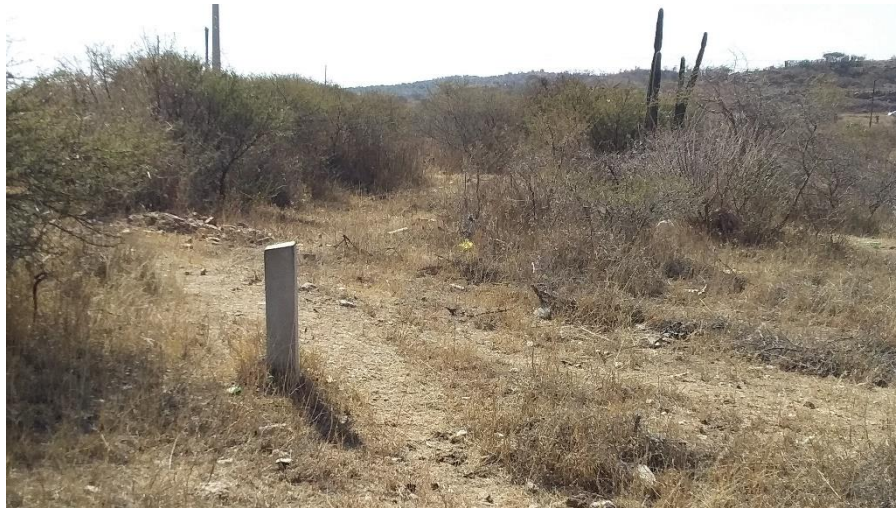
Figure 4: Pipeline marker to indicate the Lepelle Northern Water transmission in the area, situated between Alternative 1 and 2
