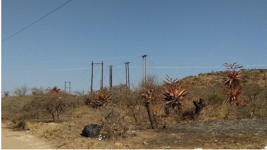
Figure 3: Existing 33kV powerlines noted from the eastern side of the proposed substation
