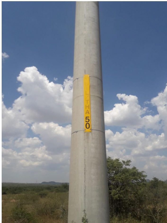
Figure 7: Existing steel monopole number 50 for the 33kV powerline, where take-off will occur for the proposed loop in loop out powerlines
