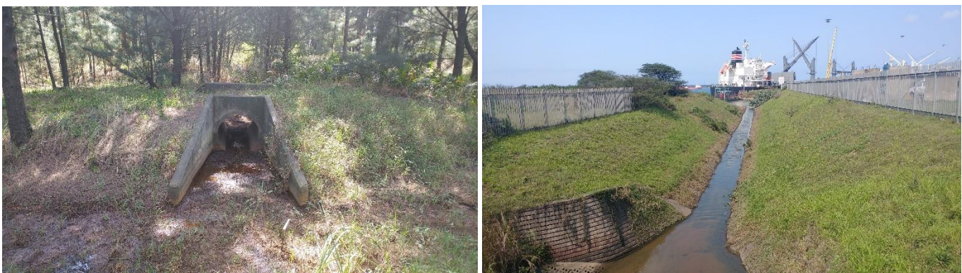
Photographs 5.4: Concrete culvert outlet from the artificial drainage channel linking into another channel within the greater drainage network (left); and the section of the artificial drainage channel exiting into the Richards Bay Port area (right).
