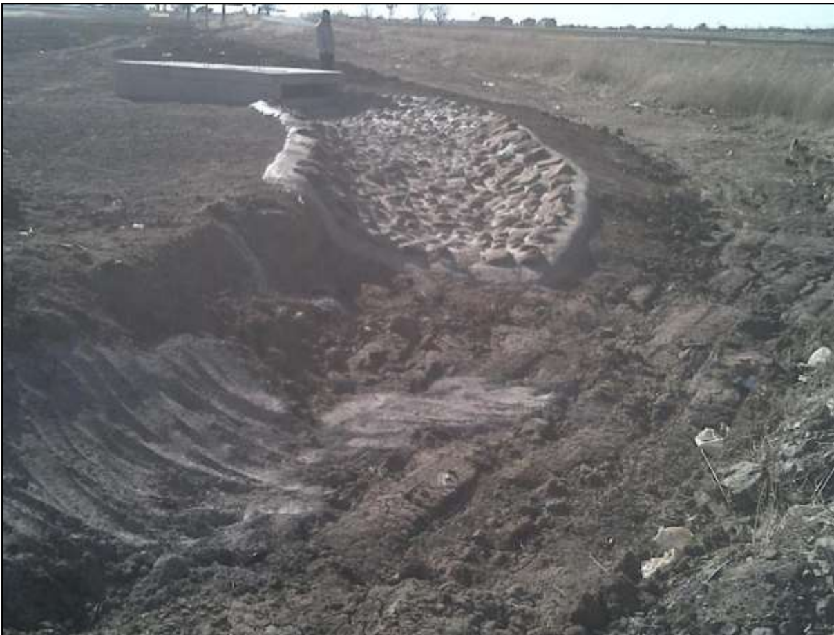
Example of the scour-pitching to be implemented where required. This is usually used to protect the environment from erosion and vegetation loss at drainage valves.
