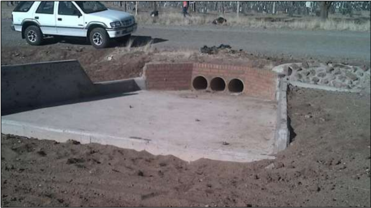
Example of a stream cross protection measured that will be implemented to protect the pipeline as well as to limit possible erosion.
