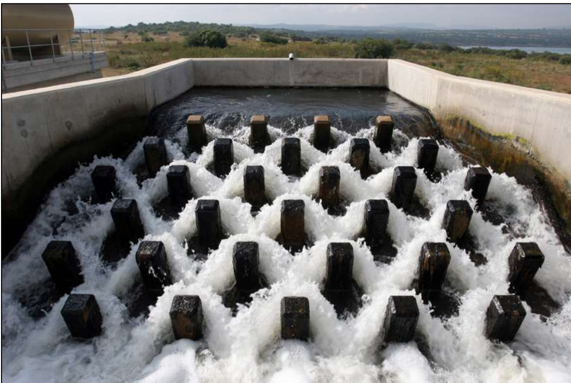
Example of the working of an energy breaker system at a pump outlet.
