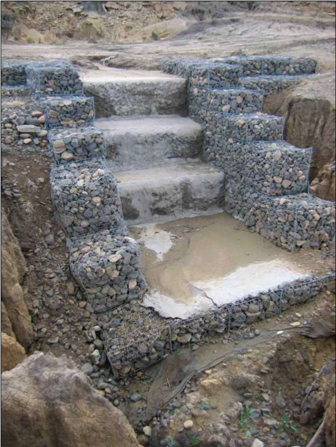
Example of a gabion constructed as part of a stream cross protection measures to be implemented
