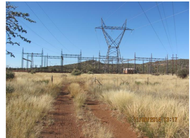
Figure 12: Steel-lattice powerline to Mangalore Substation extending from east, across Portion 4 of Farm 436 Kapstewel (Vaalkop). Note access road aligned parallel to this line.
