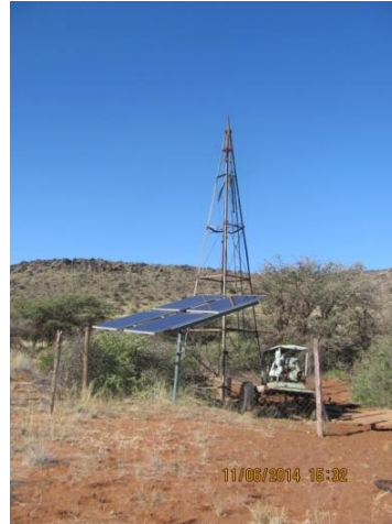
Figure 8: Solar pump and borehole.
