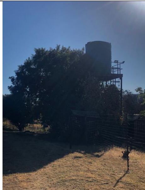
Water storage and supply to houses
