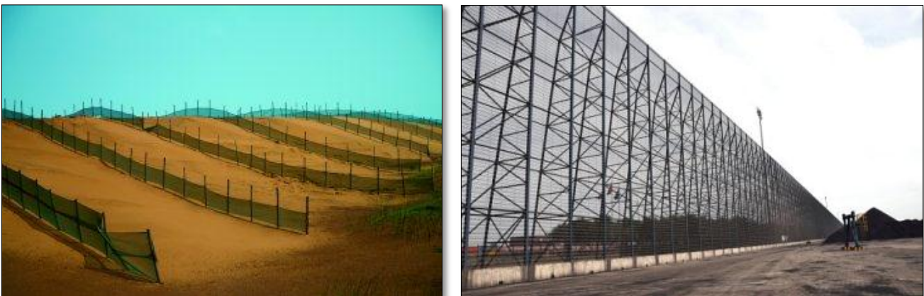
Figure 44: On-site windbreaks (left) and perimeter windbreaks (right)
