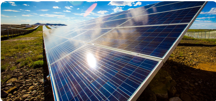
Figure 1: Solar PV facility (Courtesy of De Aar Solar)
