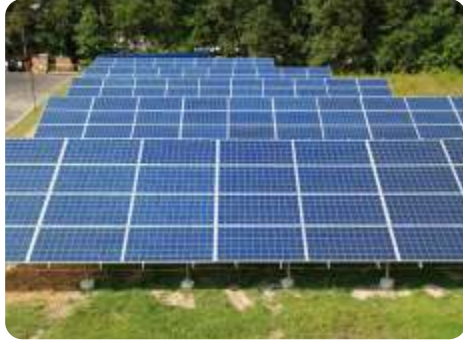
Figure 1: Illustration of PV panels (solar-energy-systems1.blogspot.com)
