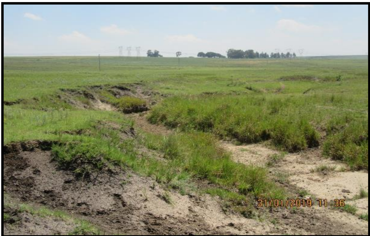
Figure 6: Evidence of in-situ soil erosion along the non-perennial stream at DCM West mine
