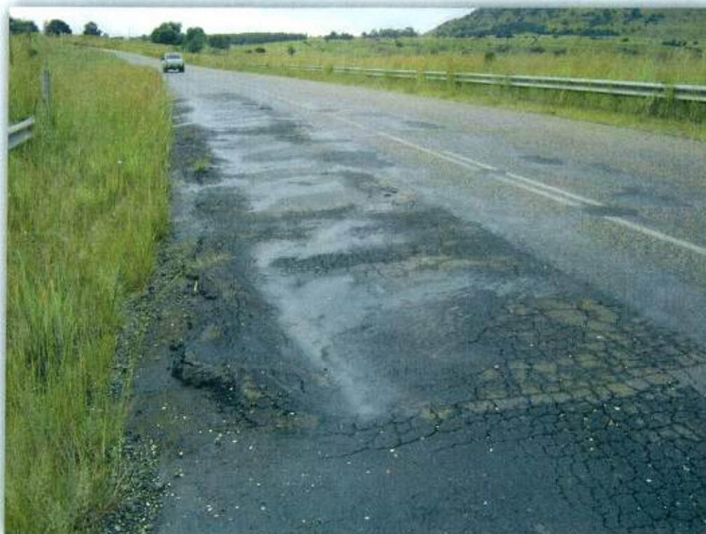
PHOTO 7: R543 Road Condition (Photo 1)
