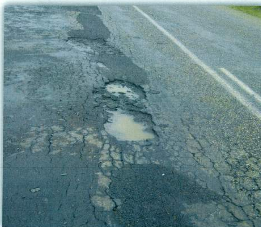
PHOTO 8: R543 Road Condition (Photo 2)
