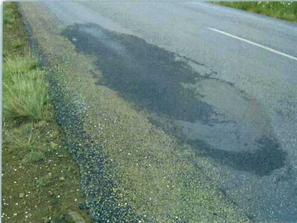
PHOTO 9: R543 Road Condition (Photo 4)
