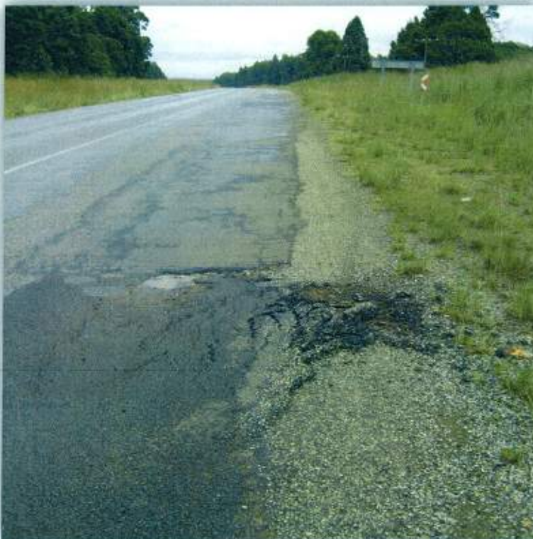
PHOTO 10: R543 Road Condition (Photo 5)
