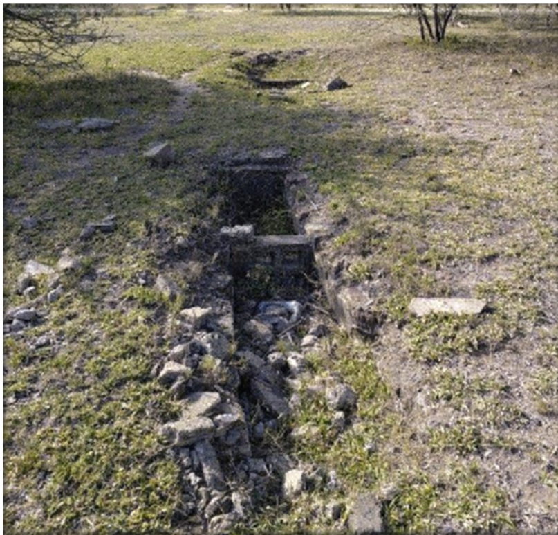
Figure 4: Degrade trough at K001
