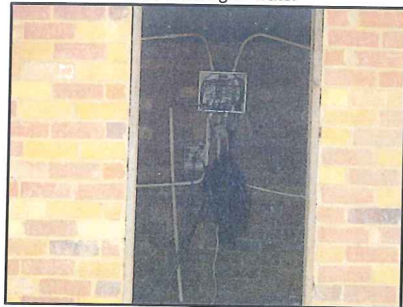
Exposed and unsafe electrical wiring
