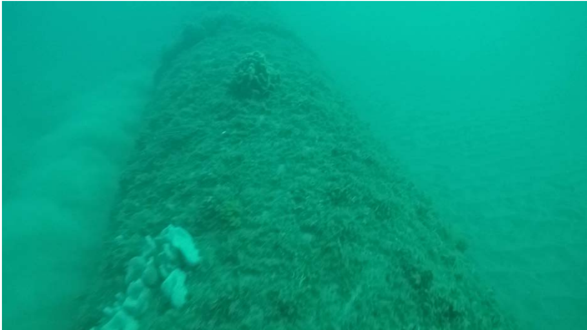
Figure 2.4 Sediment build-up is evident on the south-western margin of the pipeline and a scour moat is visible on the north-eastern margin.
