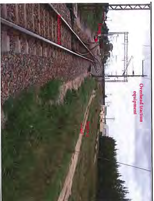
Figure 4.1 Existing loop to be extended at Barkly Bridge, Eastern Cape
