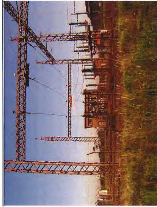
Figure 4.5 Eskom outdoor equipment (Sishen Substation)
