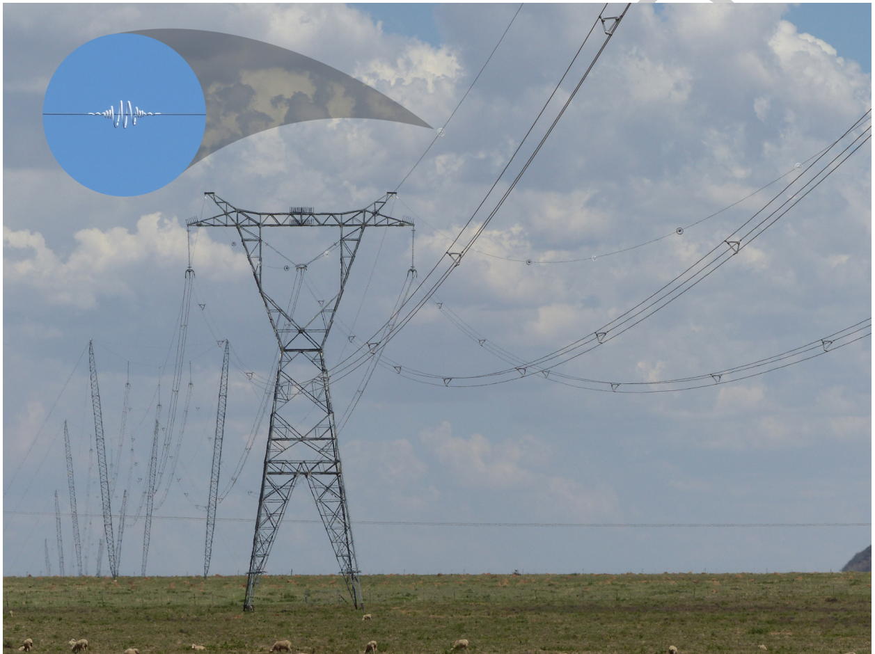
Figure 14: Example of bird flight diverters employed on the earth wires of a power line.
