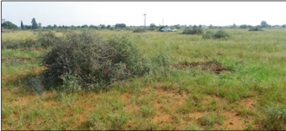
Figure 13: Bush clearance done within the north-eastern section of the development footprint area.
