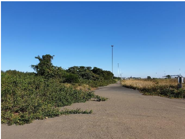
Derelict road adjacent to the unchanneled valley bottom wetland
