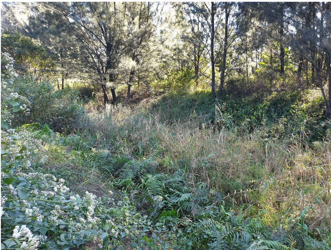
Plate 3.3. The artificial drainage channel showing clear channelling and invasive Pine trees along the channel edge.
