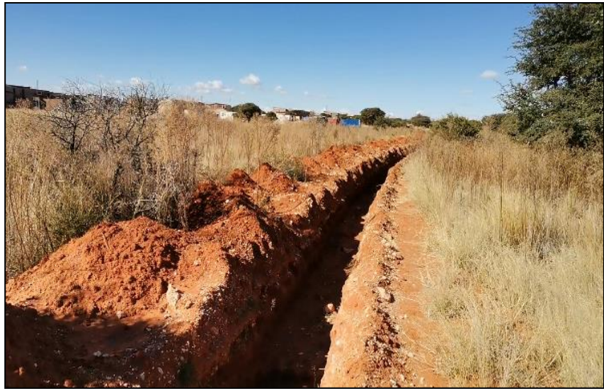
Figure 7 An open trench 50-70cm deep, running across VU-E. The first phase of student accommodation is visible in the background.
