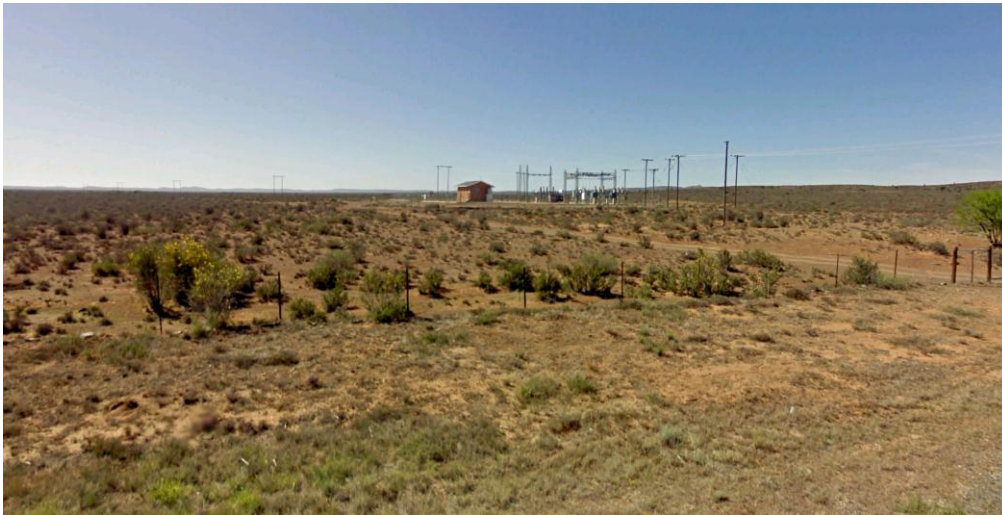
Figure 7: Photograph illustrating the substation on the project site. The planned PV/CPV 'strings' are to be established around the substation.
