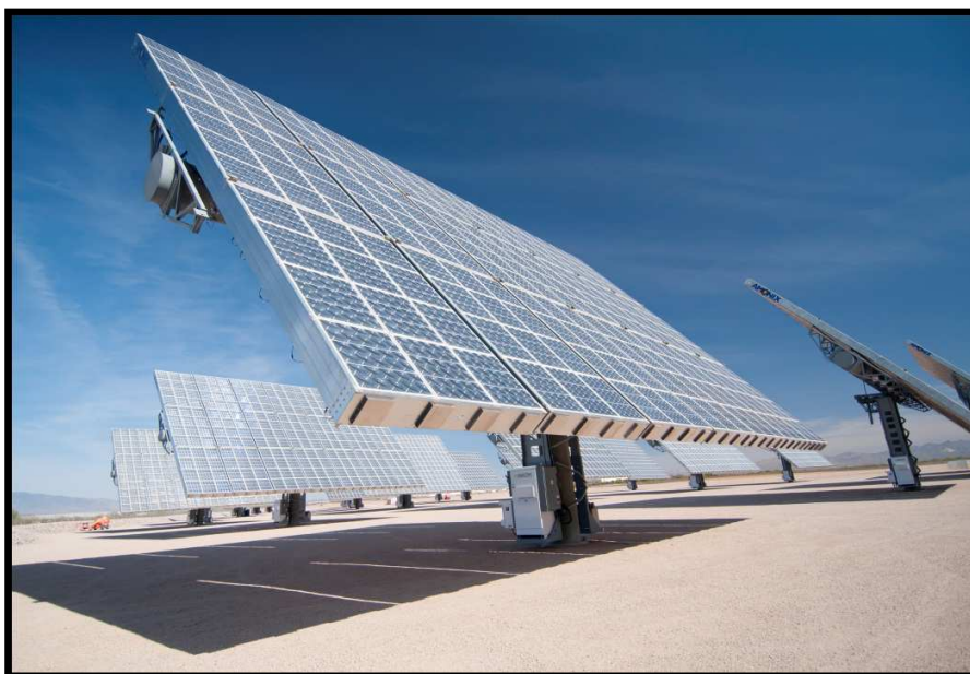
Figure 1.5: Example of a CPV plant (Source: Savannah, 2012)
