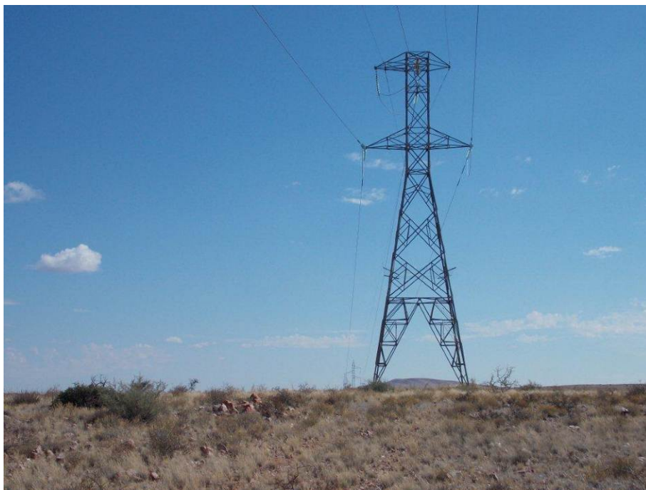
Picture 3: Existing Gordonia/ Garona 132 kV power line
