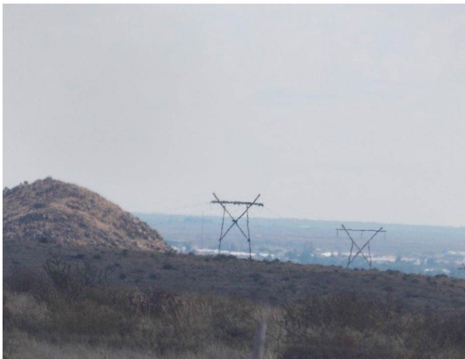
Picture 4: Existing Gordonia/ Kleinbegin 132 kV power line
