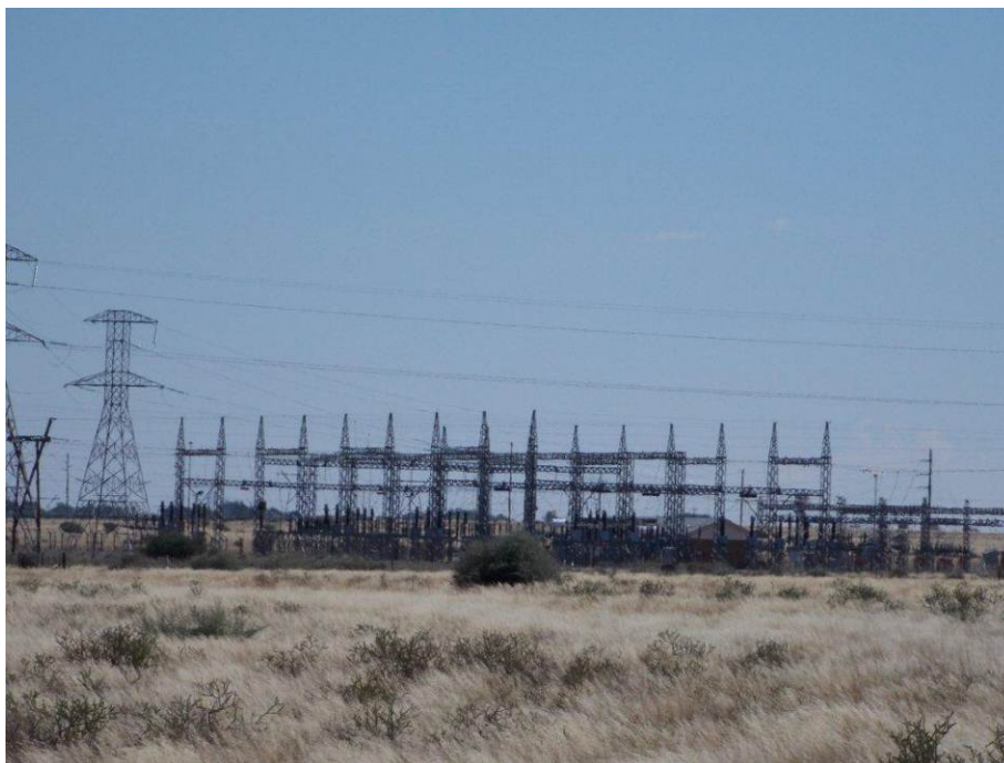
Picture 5: Gordonia substation
