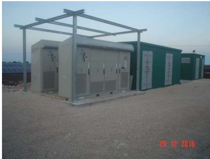
Figure 15 : Typical on-site substation
