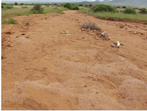
Figure 37: Even in the flat areas the velocity and cumulative effect from run-off result in increased erosion.
