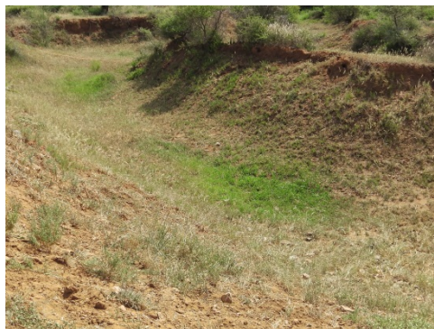
Figure 42: Erosion gullies associated with increased run-off from hard surfaces.
