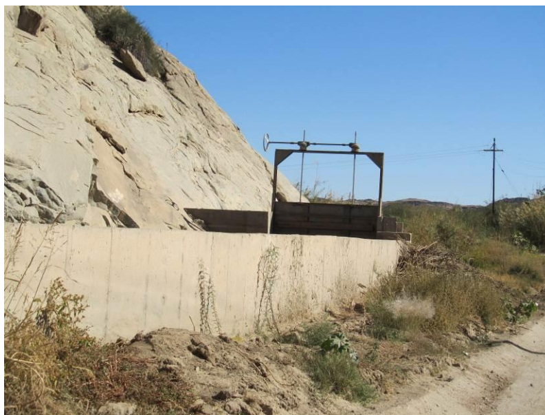
Figure 10: Irrigation distribution canal in the area of the newly proposed abstraction point
