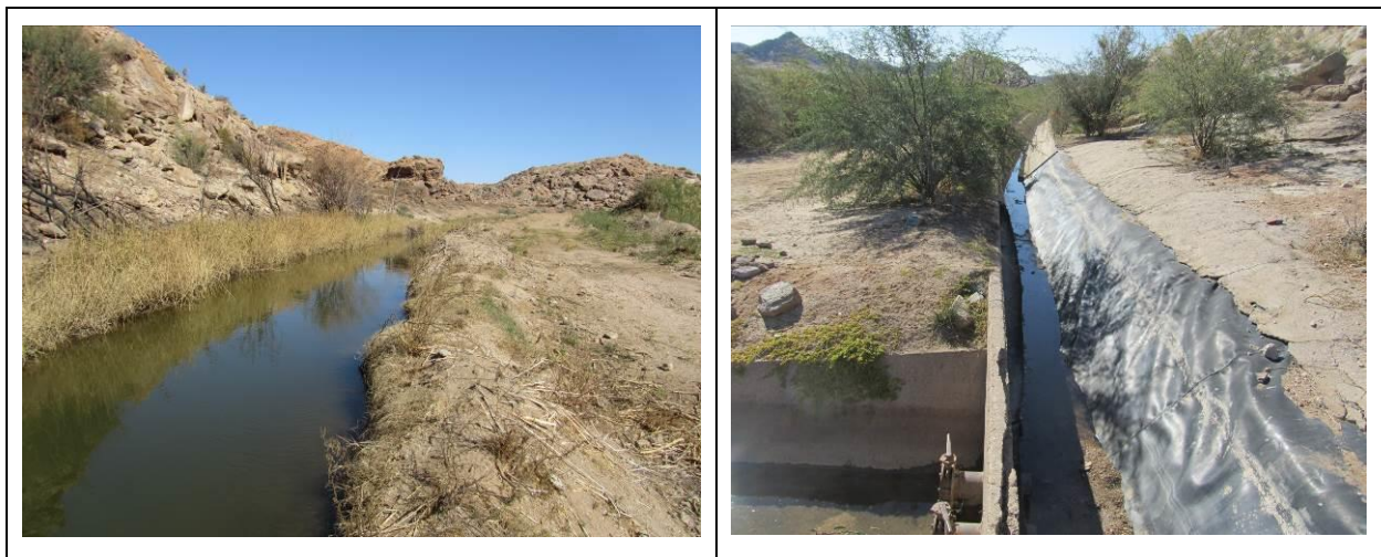
Figure 5a and b: Earthen canal and plastic lined canal at the end of the distribution system
