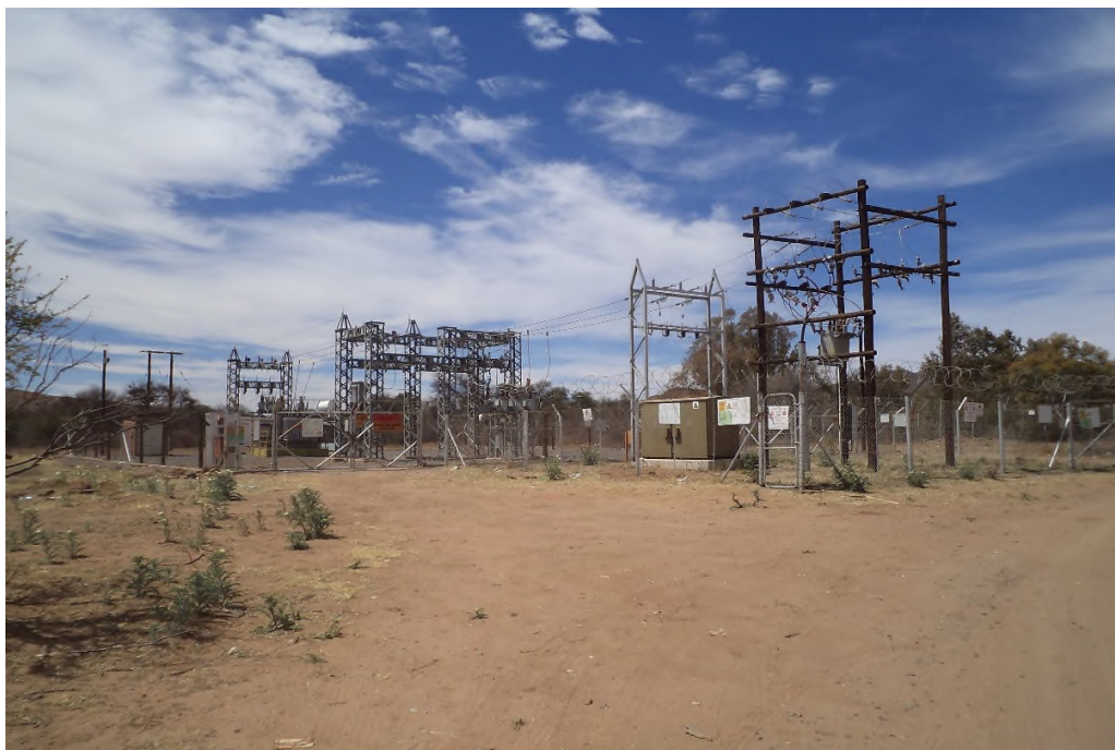
Figure 18. The existing Olifantshoek Substation in the town of Olifantshoek
