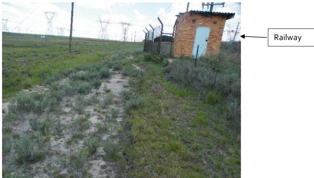
Photograph 1: The existing substation and powerlines at the project area
