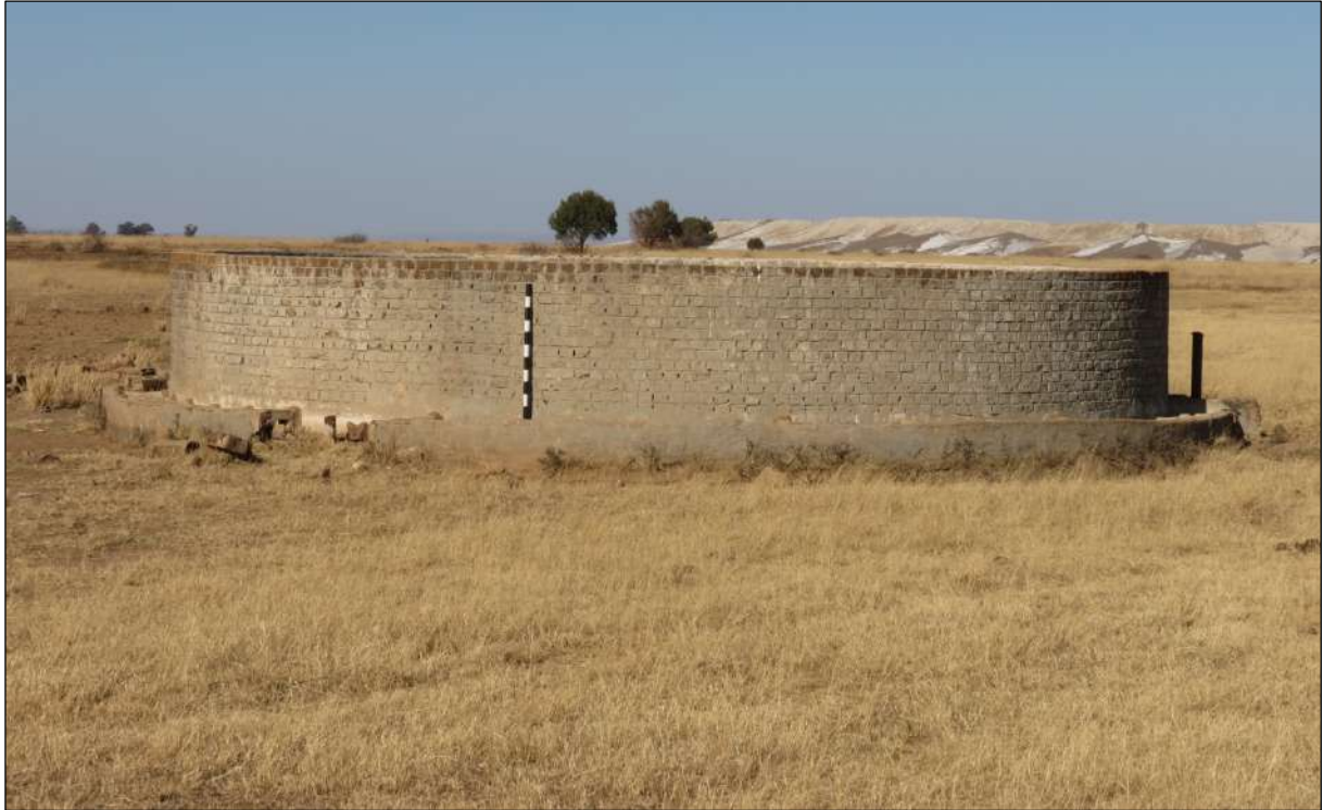
Figure 38 – General view of the brick-built reservoir at site AGA-MWS-WBP-2. The existing Kareerand TSF can be seen in the background on the right. Scale is in 10cm increments.
