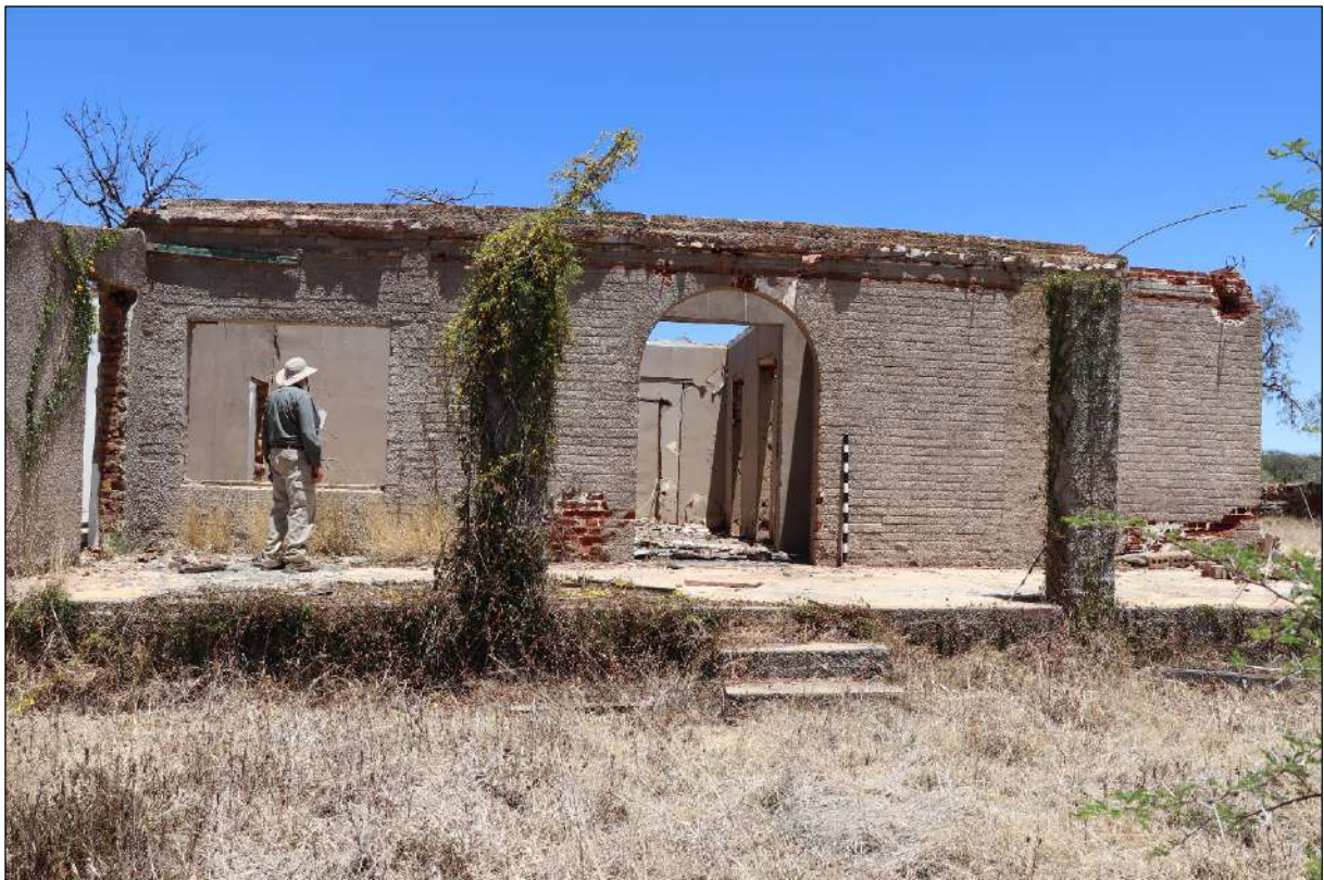
Figure 86 – Eastern façade of the farm dwelling identified at site AGA-MWS-UMF-3. Scale is in 10cm increments.
