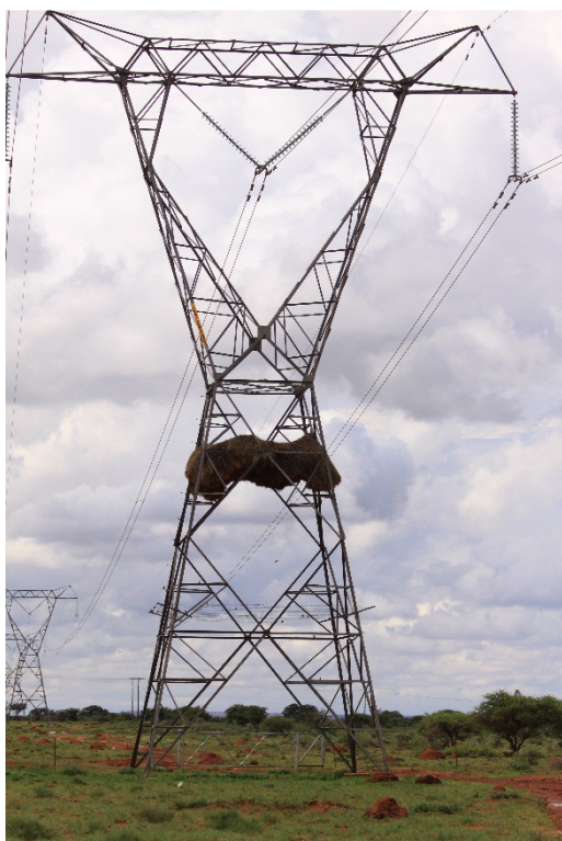
Figure 11: Sociable weavers utilizing the power line tower structures for the construction of their nest.
