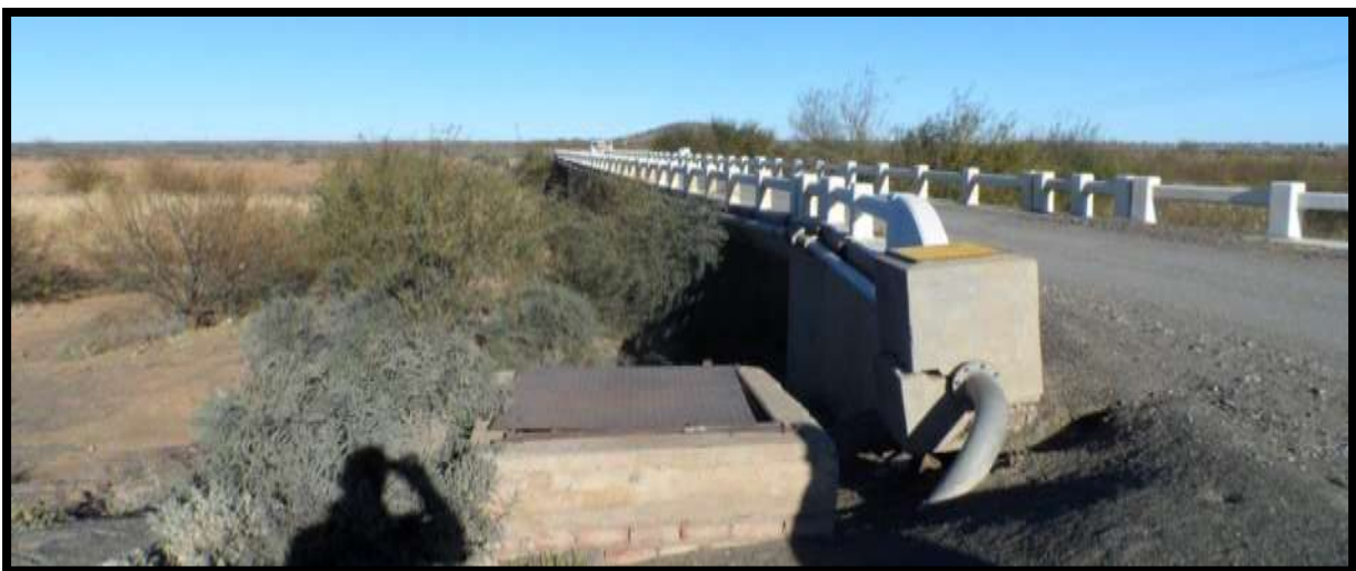
Photo 7: Bridge over the Sak River, showing the location of the existing pipeline attached to the bridge
