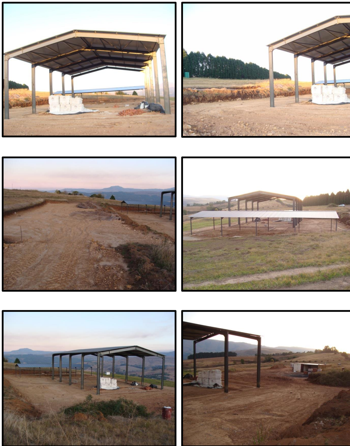
Figure 5-10: Several terraces had been cut into the slope of the mountain, with two partially built shed-like structures erected on the largest of these clearings. An adjacent terrace on a higher level was in the process of being levelled out and stones were being added for flooring foundations (Fig.7). The lower terrace extended to the west of the two built structures where some shipping containers had been placed for equipment storage (Fig.10). The exposed walls of red sediment created by the cutting revealed a stratified upper soil layer which did not appear to contain any archaeological material. Fossil-bearing rock had been used as a foundation to strengthen the floor of the terraces, so another rock type will have to be used to finish the remainder of the flooring for this development
