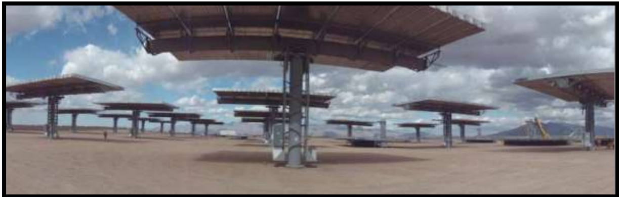
Photo 6: Typical layout of such a solar site (Image courtesy of Amonix, a leading designer of CPV technology)
