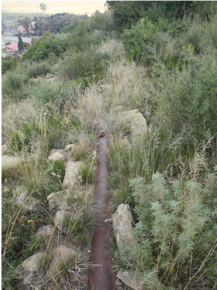
Figure 7: View of an existing pipeline along the slope of the hill. The current proposed pipeline should be installed along the same method where with regards to the sandstone hill, i.e. on top of the soil surface or semi-imbedded.
