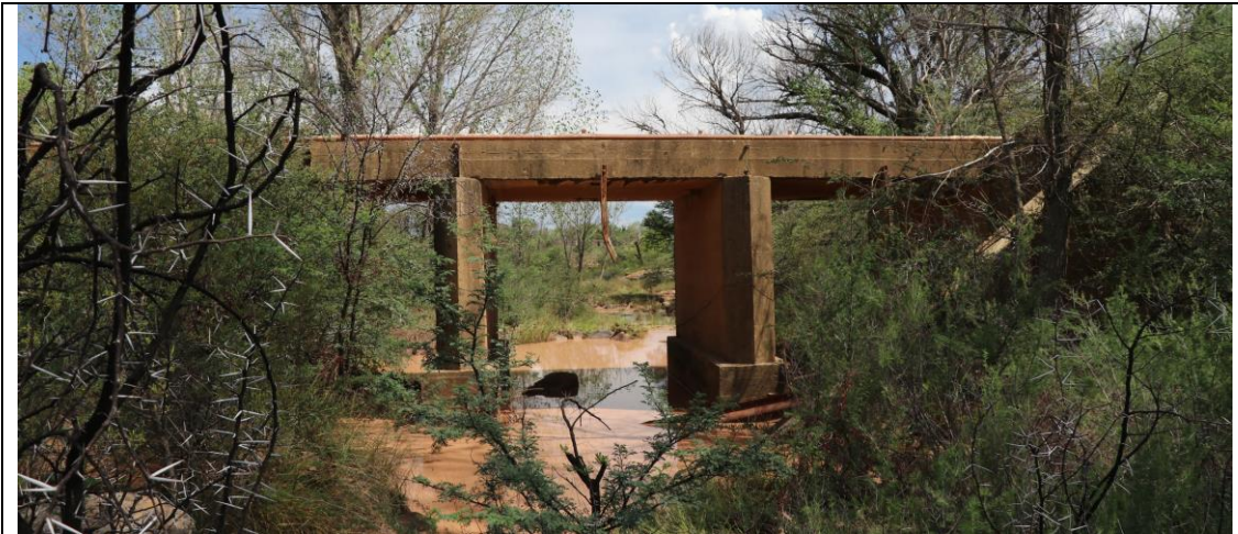
View of the gravel road and bridge over the Sandspruit. This will clearly have some impact in terms of flooding and scouring.
