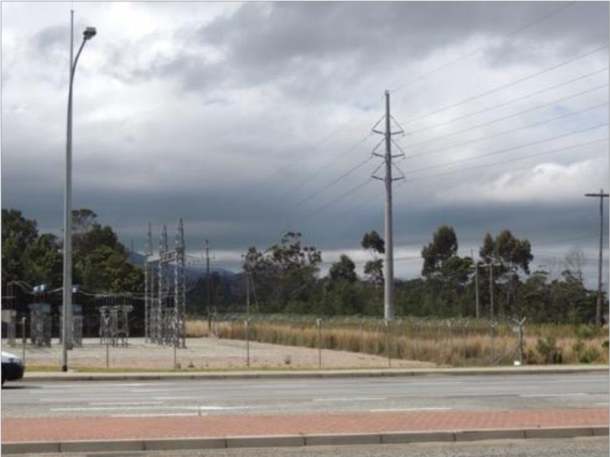
Figure 3: Example of transmission lines link to a small substation (Source: VRMA)
