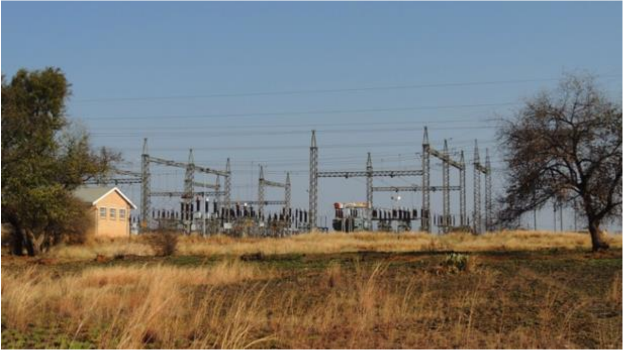
Figure 8: Photograph of the regional Eskom Substation
