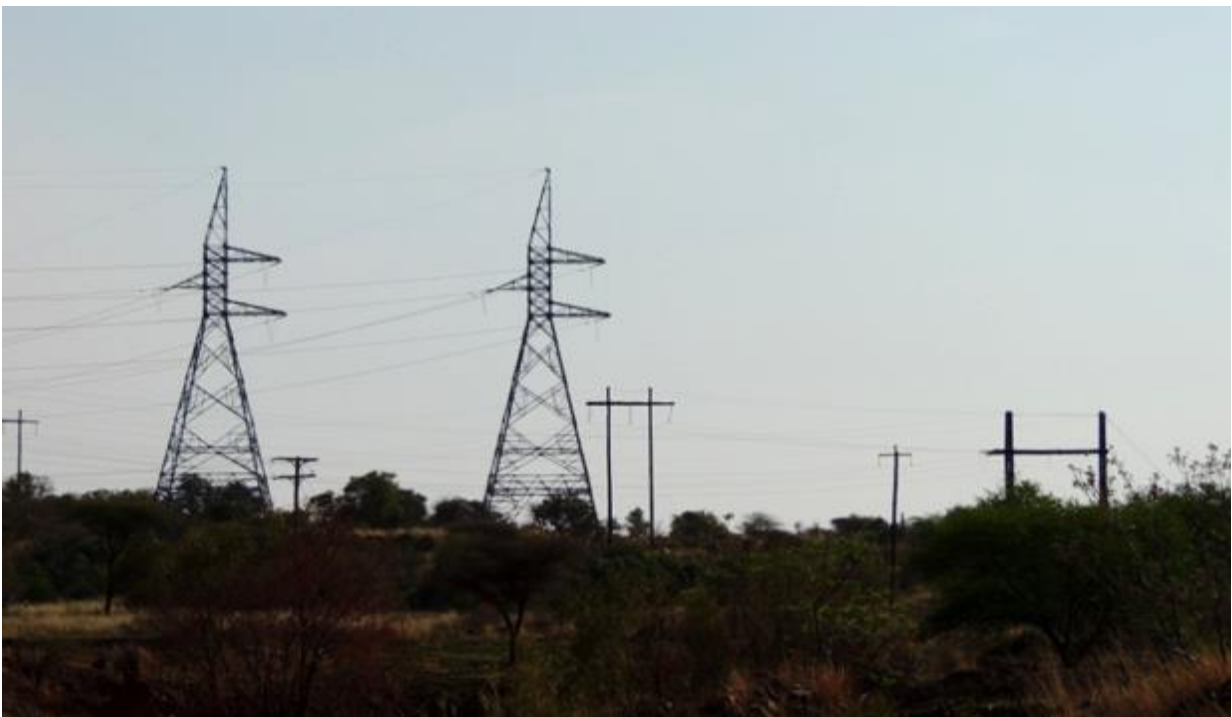
Figure 9: Photograph of the existing Eskom power lines routed to the south of the proposed corridor.
