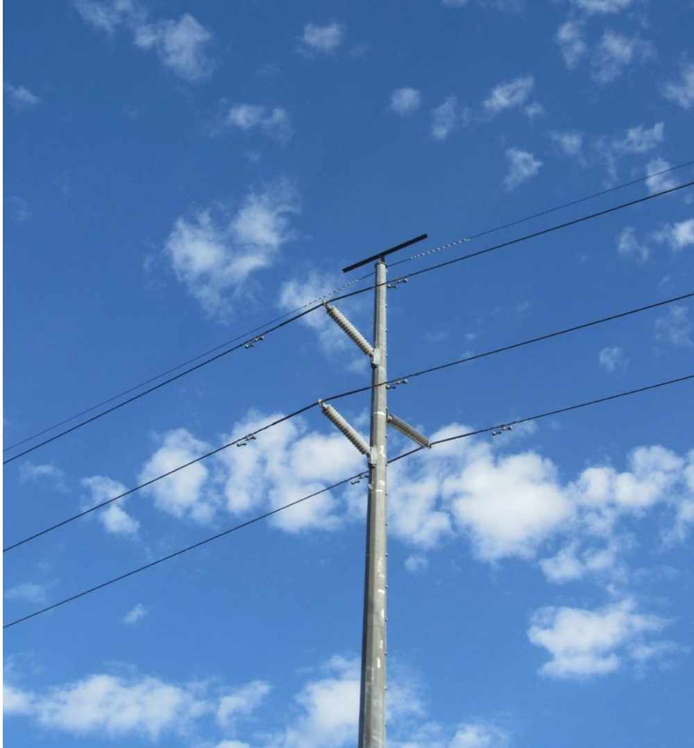
Figure 7: An example of a bird friendly monopole, adapted with bird perch, currently used for several of the existing lines around Watershed sub-station.
