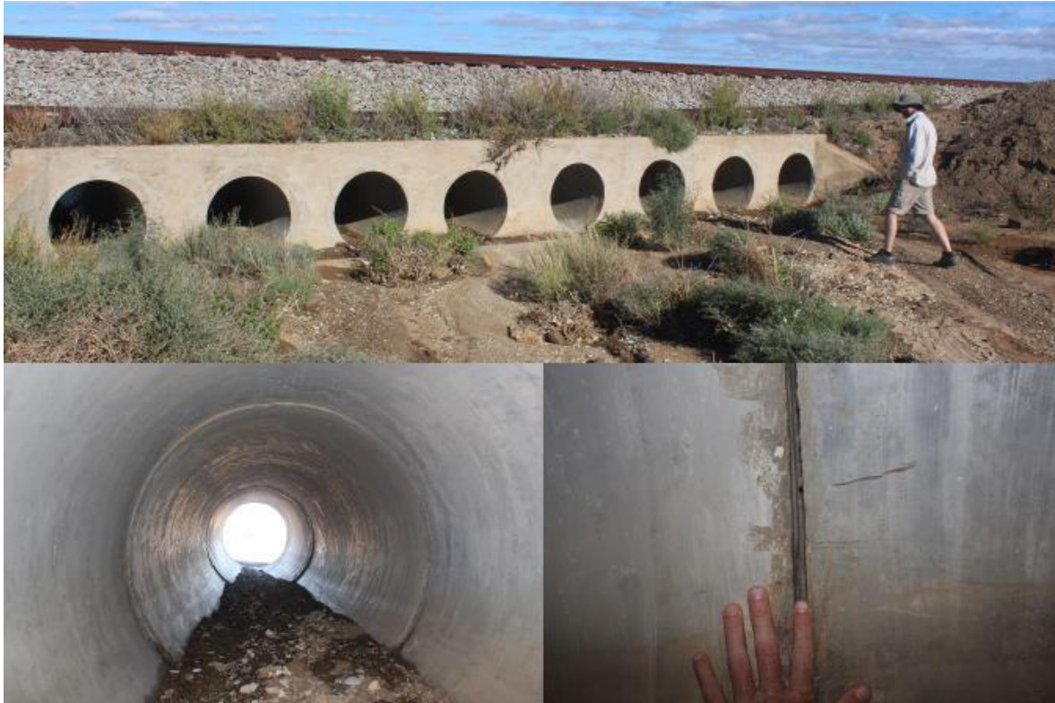
Figure 3-19: Photographs of the railway water underpasses and features relevant for potential bat roosts.
