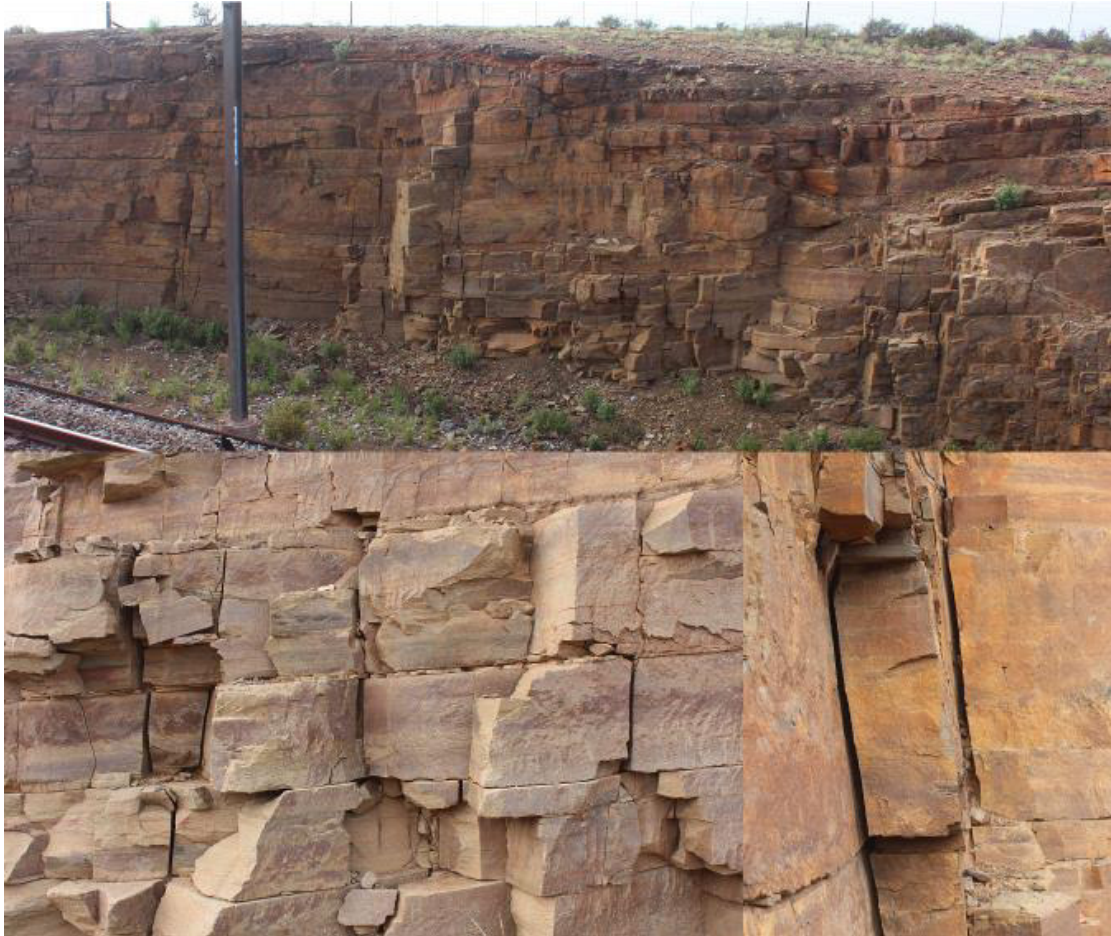
Figure 3-22: Photographs of the railway in-cut banks showing crevices relevant for potential bat roosts (LR4).
