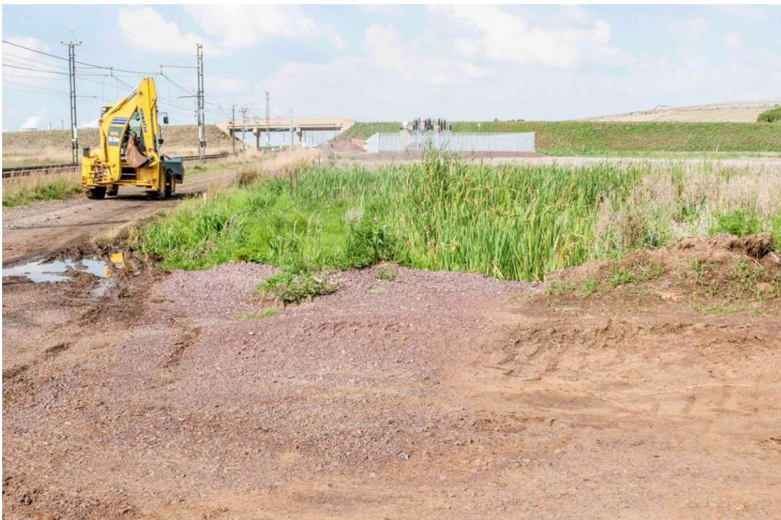
Figure 4: The railway line and service road. Photographed at the site where the new substation is being constructed.
