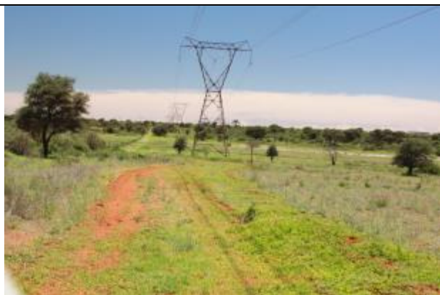
Photo 8: Service road of the 275kV line, crossing the Ga-mogara watercourse.
