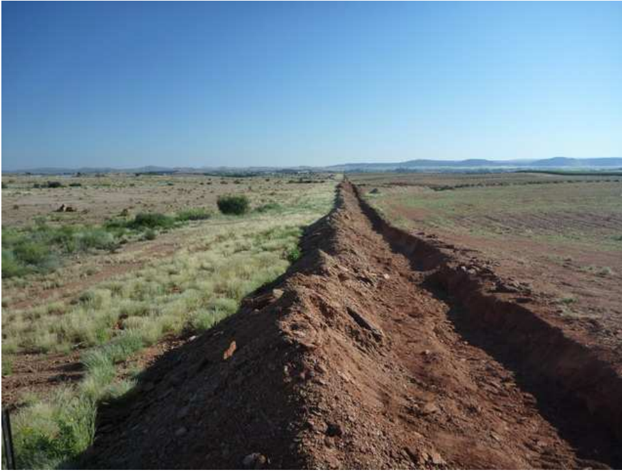
Figure 9 Prepared soils (ripped and levelled) on the eastern side (right) of the site and original soils on the western side (left)
